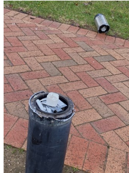
Park light broken by vandals
