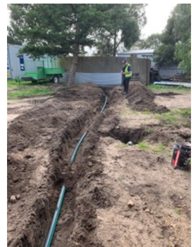
Pipe for the fire hose
