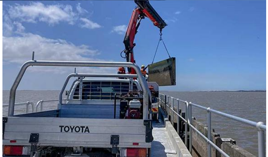
Removing concrete stop logs from the barrages, allowing water to flow between the lower lakes and Coorong areas.
